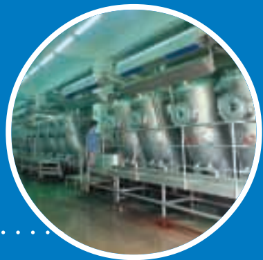
8,000-pound Dyeing Tank
